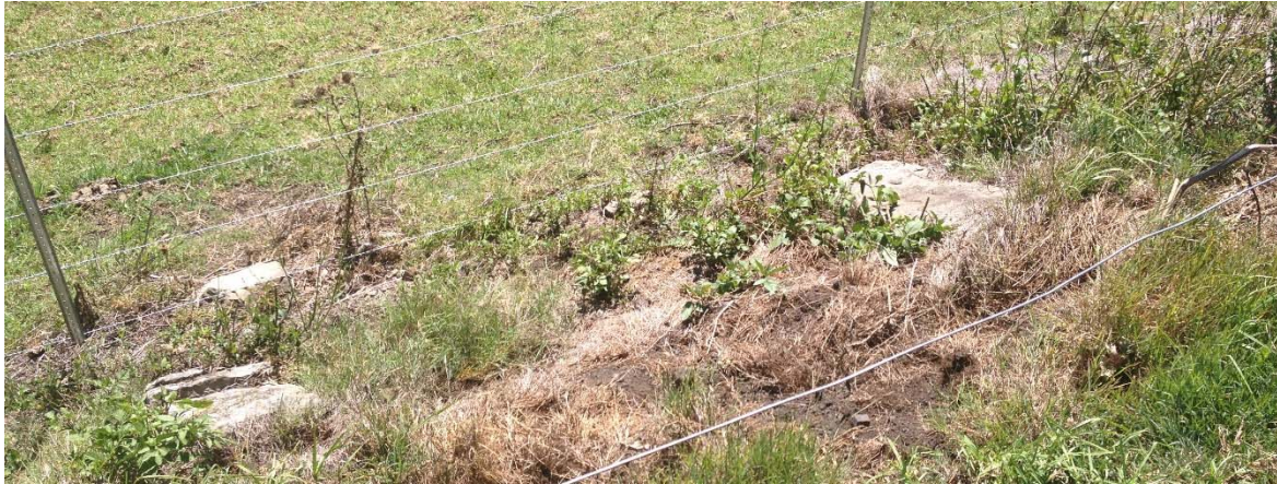
Photo 4: Sandstone blocks along the battered slope of the northern boundary The eastern paddock, which is approximately double the size of the western paddock, also appeared to be benched. There were a number of patches of bare soil or sparsely vegetated within the eastern paddock. These appeared to contain fill material comprising of gravel, coal, charcoal and crushed concrete (Photo 5).
